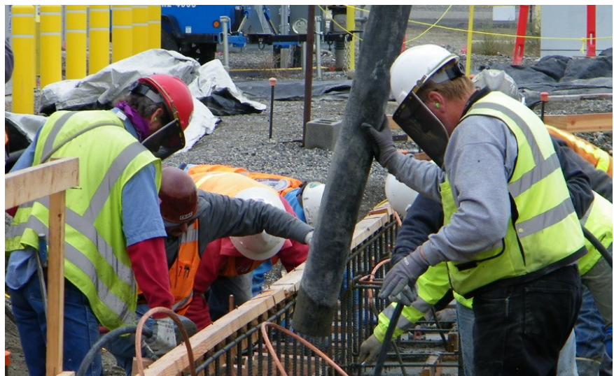
Concrete placement for the K West Annex building that will house the sludge retrieval equipment.
