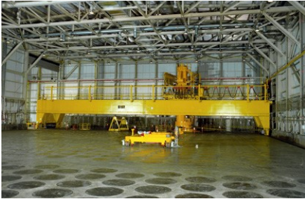
A crane inside the 42,000-square-foot Canister Storage Building is used to lift multi-canister overpacks from below-grade concrete vaults.
