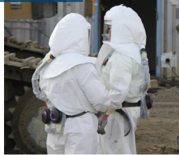
Workers near the demolition activities wear protective clothing and breathe filtered air.
