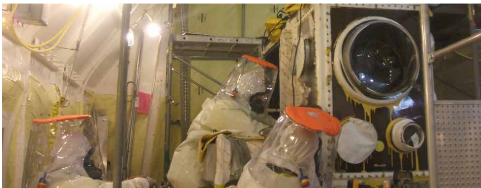
Employees cut apart and remove the most hazardous glove box, which is a large, contaminated enclosure once used to handle plutonium.
