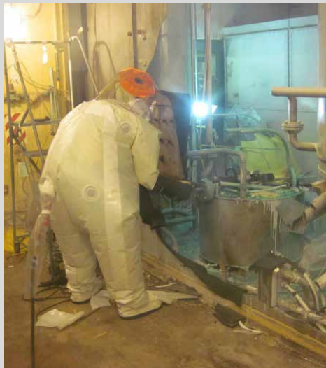
A worker dressed in multiple layers of protective clothing prepares chemical tanks for removal during demolition.
